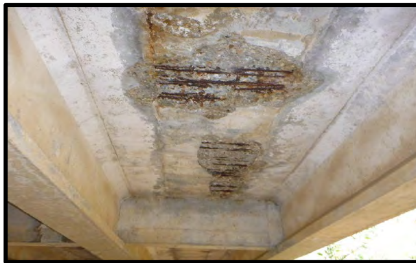
Exposed and corroded rebar in closure pour between "T" girders
