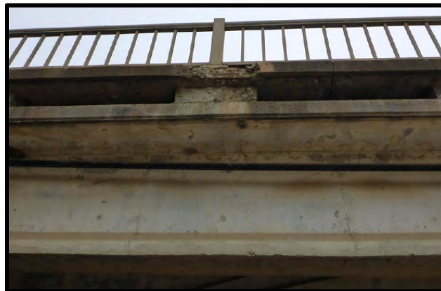
Image showing baluster bridge railing and spalling concrete
